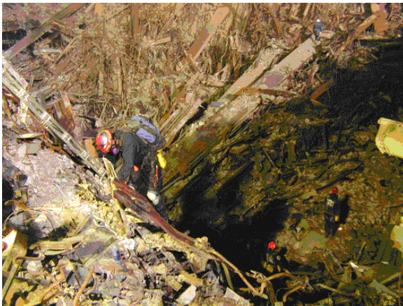
Figure 9-3 - GZ workers descend into the subbasements below WTC2. While there is extensive damage, there is little building debris at the bottom of the hole. There is no
